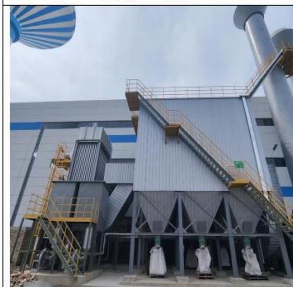
SNCR+急冷+表冷+石灰石脱硫+活性炭喷射 +布袋脉冲除尘
